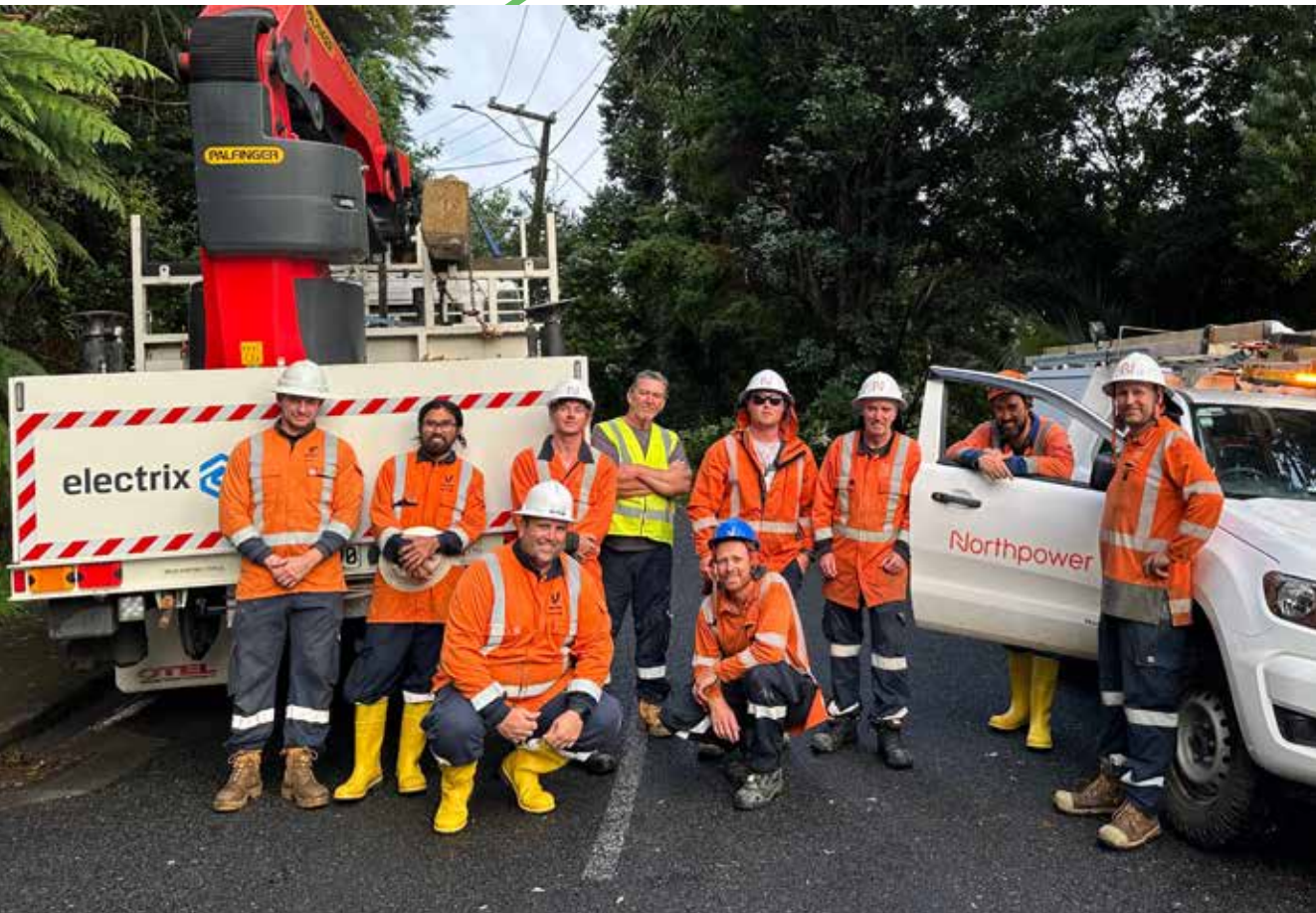
Omexon (formerly Electrix) and Northpower crews work day and night to keep the power on for Vector customers.
