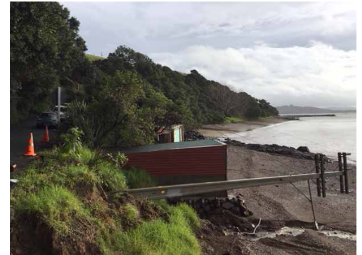
Road slips causing a power line to fall over at Kawakawa Bay
