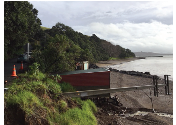
Road slips causing the line to fall over at Kawakawa Bay
